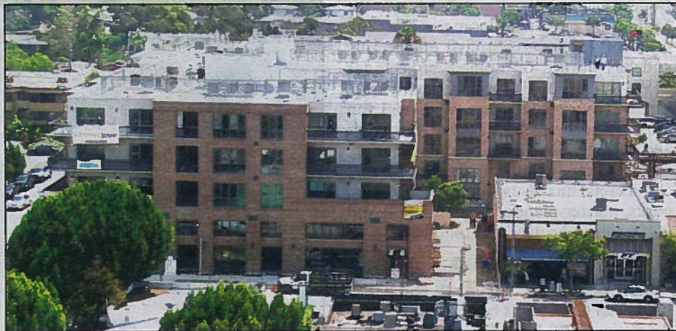
Photo courtesy of Barbara Metz/Metz Public Relations Construction has reached the 80 percent mark for the 120,000-square-foot residential/retail mid-rise at 1Mission in the heart of San Diego's Mission Hills.
